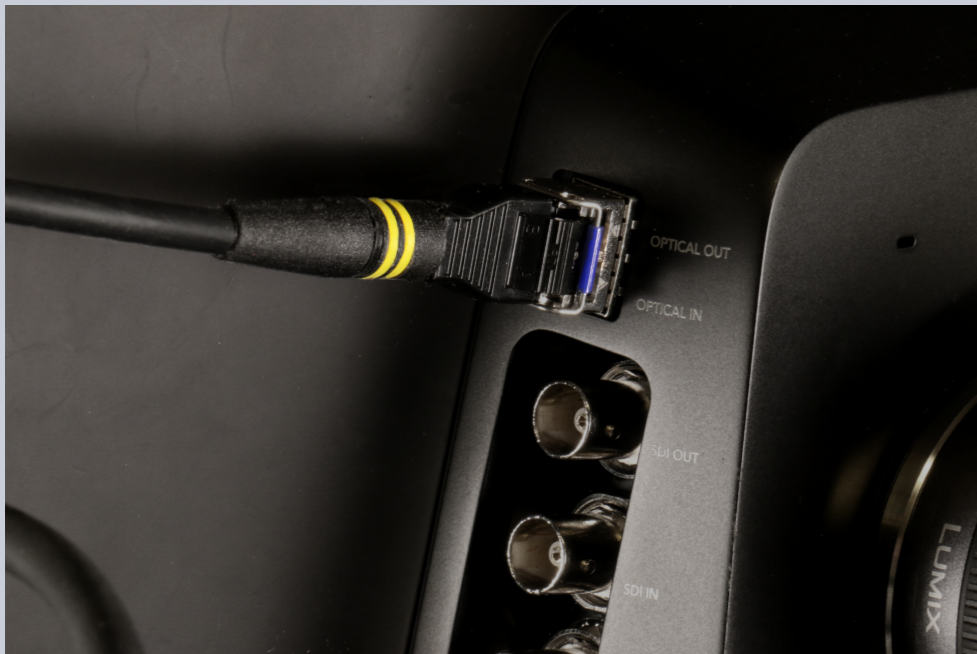
LC Duplex bridging cable ending in the SFP of Studio Camera
